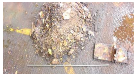
Over the course of the survey, huge amounts of scale and dropped objects were removed.
