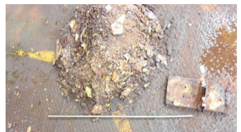
Over the course of the survey, a significant quantity of scale and dropped objects were removed.
